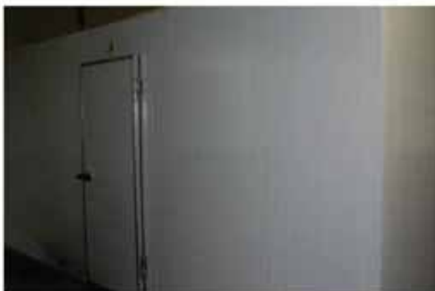
Walk-in cold room and freezer
